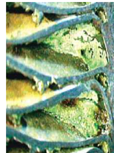
Figure 8.30 (a) General copper corrosion.
